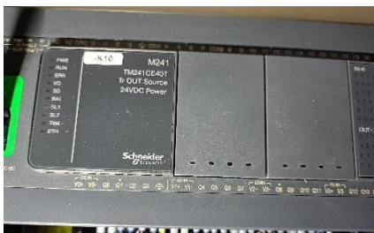
SB-106: PLC for controle box
